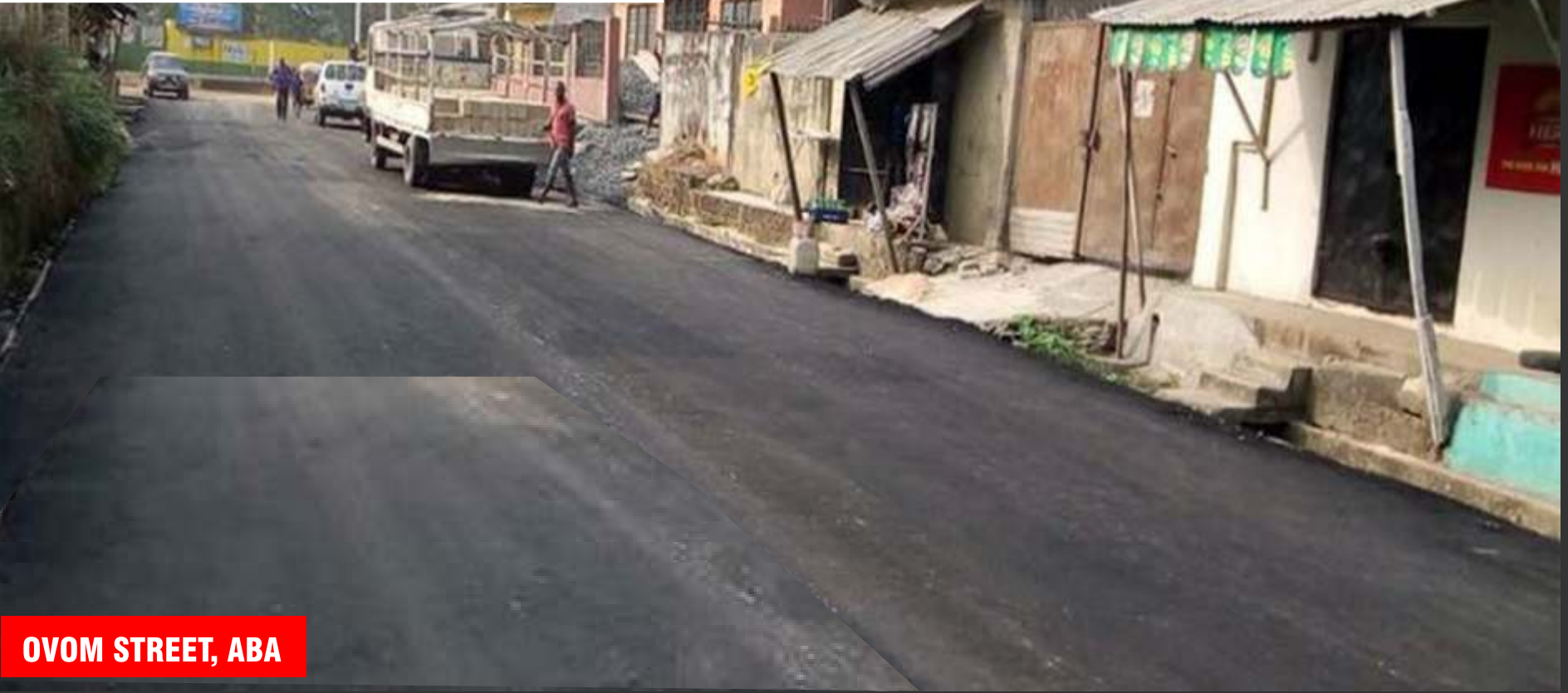
OVOM STREET, ABA BEFORE
